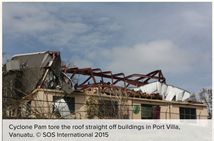
Cyclone damage in Port Vila. © SOS International 2015
